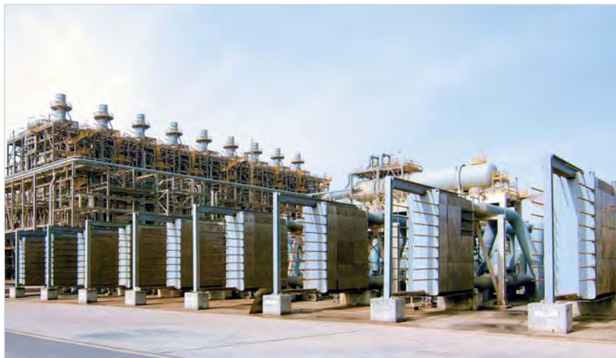
SPX APV plate heat exchangers at Ras Laffan, Qatar. Photo courtesy Ras Laffan Olefins Company (RLOC)
