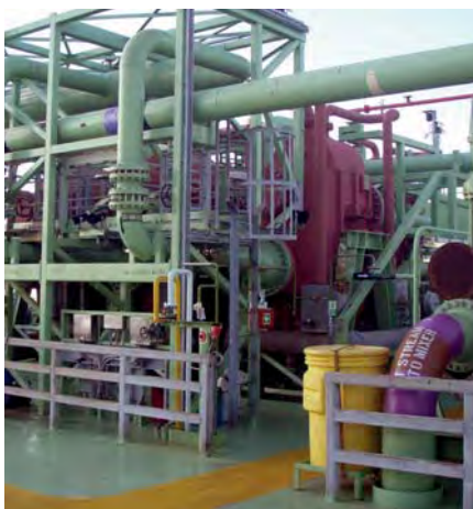
APV Hybrid welded plate heat exchangers operating as wet crude heaters on board BW Offshore FPSO Yüum K'ak'Náab in operation for Pemex. Photo courtesy BW Offshore.
